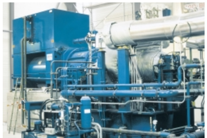
Fig. 19: BHS E-PACK® Epicyclic Gear Unit mounted on the generator, driven by a steam turbine.
